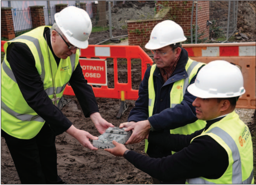
FEBRUARY 2025: The growing Catholic community of St Philip Howard Parish took another significant step forward in its ambitious £3 million redevelopment project as Bishop Peter Collins blessed the foundation stone for the renewed church.
